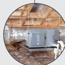
Indoor Fan Coil Unit (Installed within roof space)
